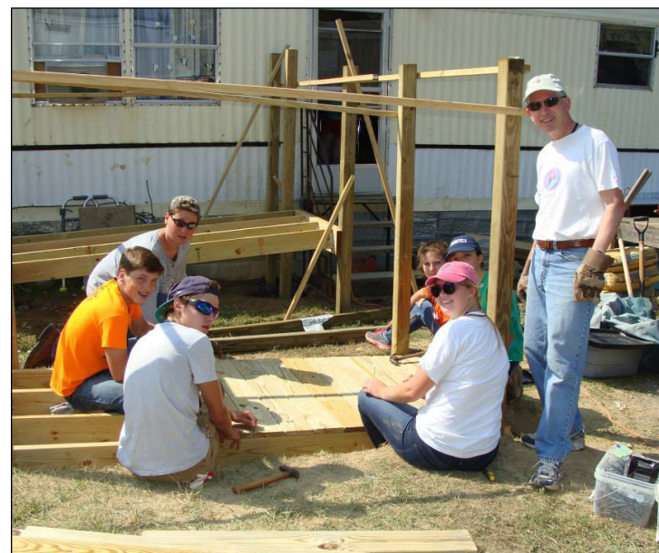
Building wheelchair ramps is one of the campers' favorite projects. This team worked diligently and accomplished more than planned.
